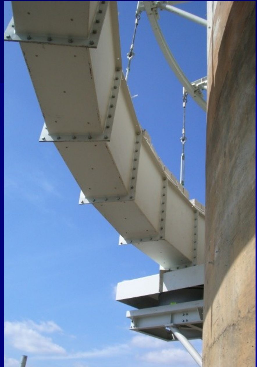
Fig 6 : view of one of the 5 damping units
