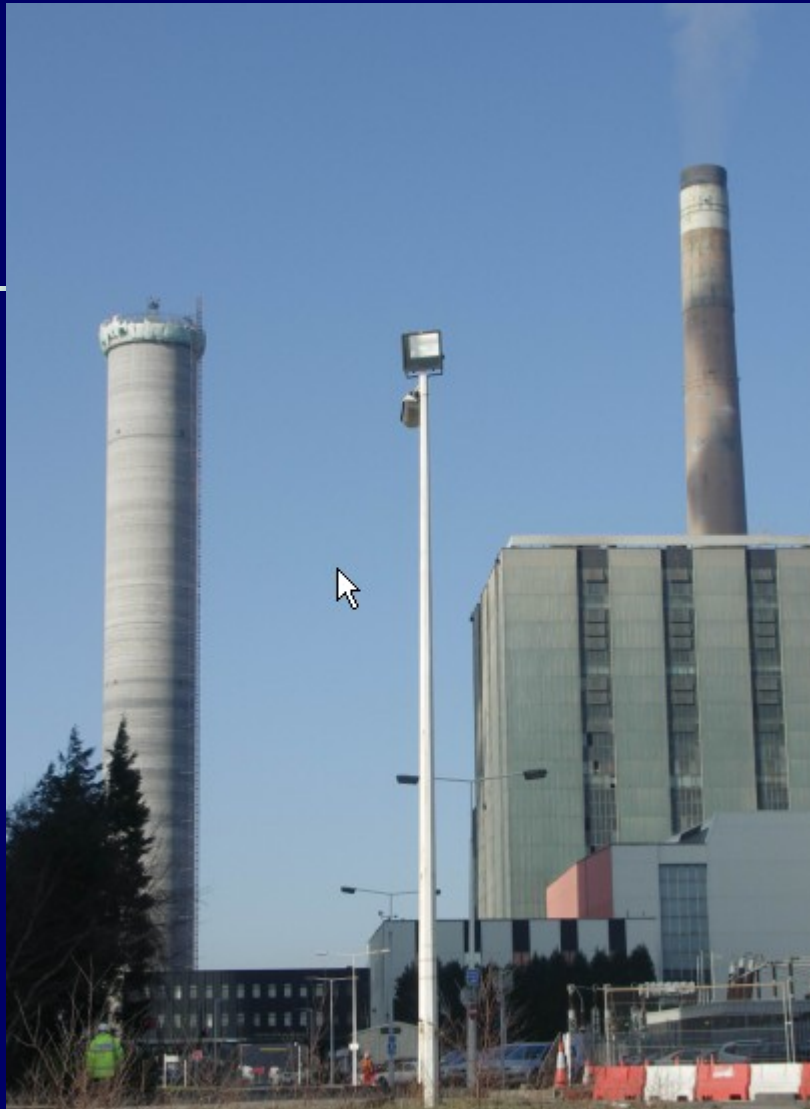
Fig 2 : new concrete stack under construction at 110 m from the old concrete stack
