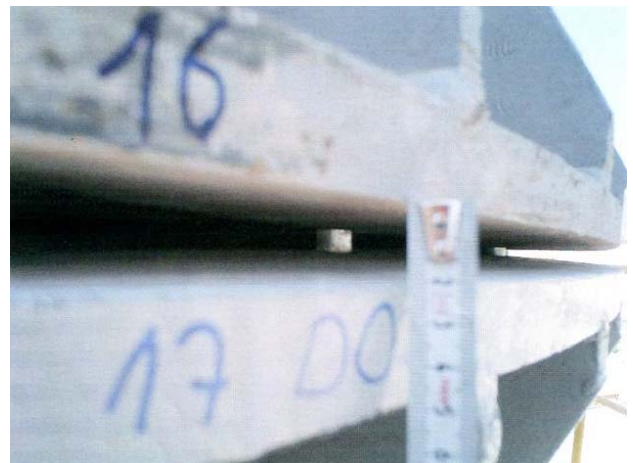
Fig 8 : gap in a flange assembly
