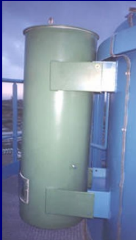
Figure 28 : Horizontal Tuned Mass Damper enclosed in a box
