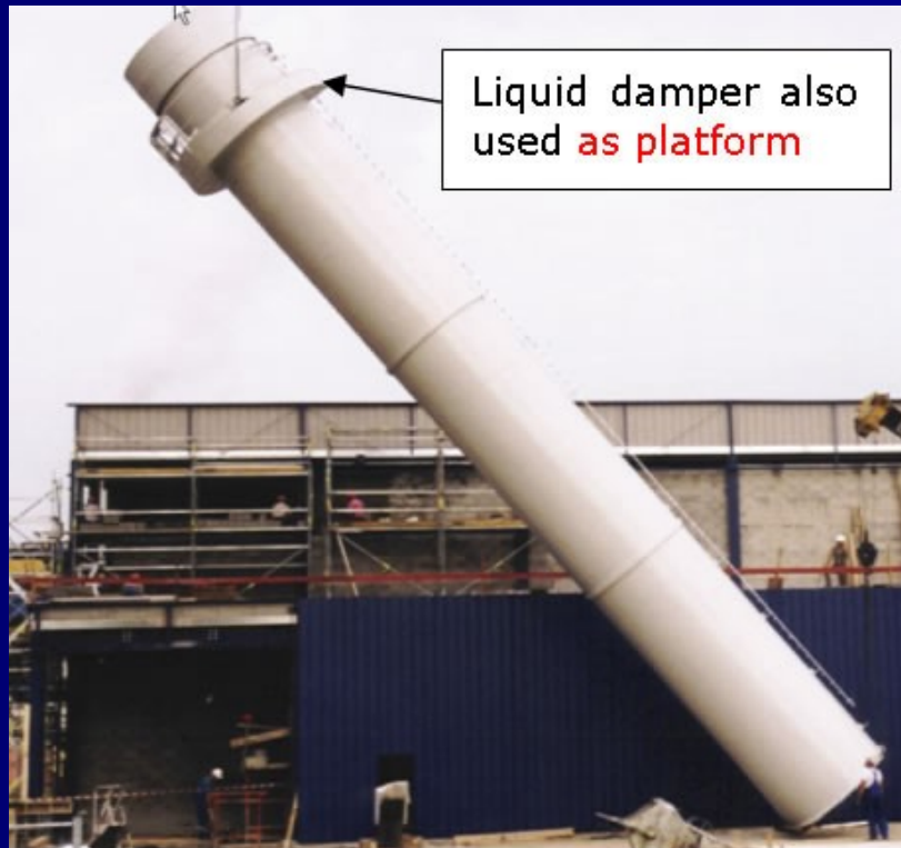
Figure 26 : steel stack with a liquid damper used as a top platform
