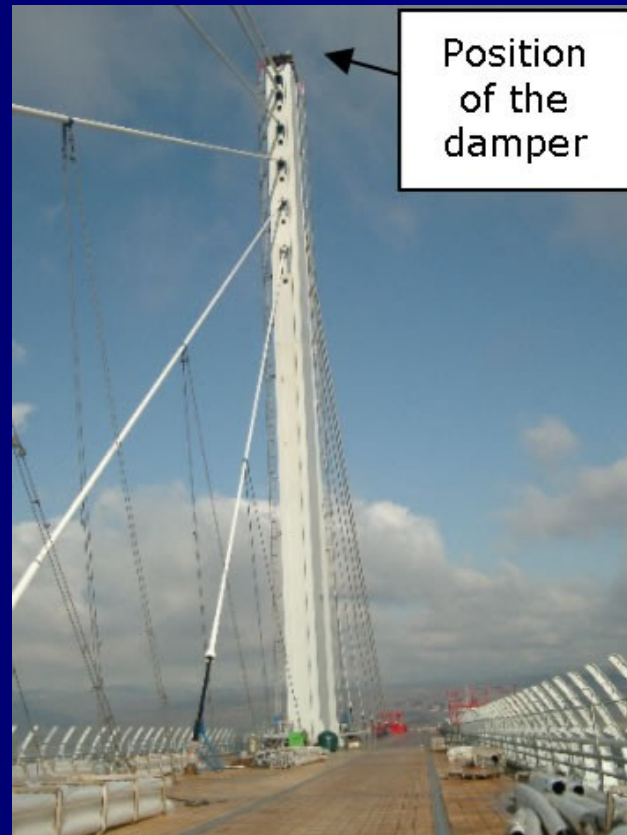
Figure 34 : detail of the steel mast damper- to be installed at the top
